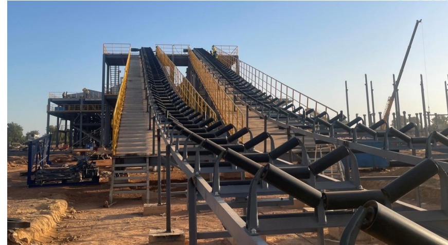
Dual module crushed ore feed conveyors
